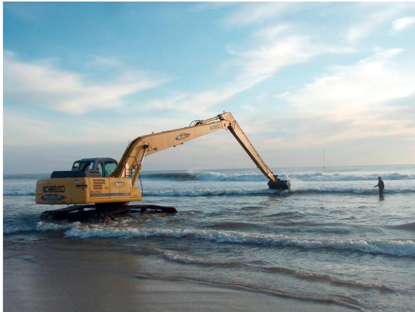
Figure 1. Backhoe excavating a hole in the inner surf zone near Duck, NC, at low tide.
